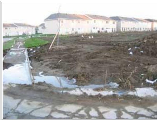
Figure 6. Exposure of soil at a construction site creates potential for soil erosion by water, wind, or both. Eroded soil pollutes waterways and causes sedimentation of ponds and reservoirs. Image courtesy of Tim Kettler
